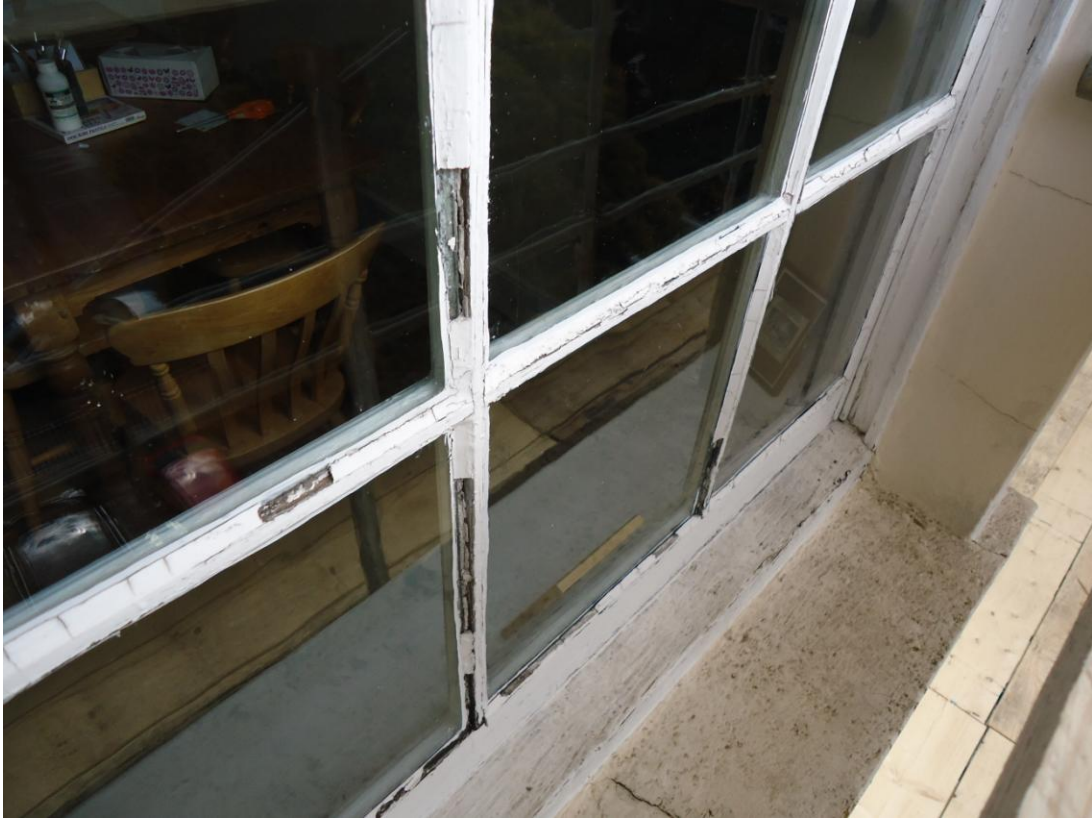
Example of failed putty lines
