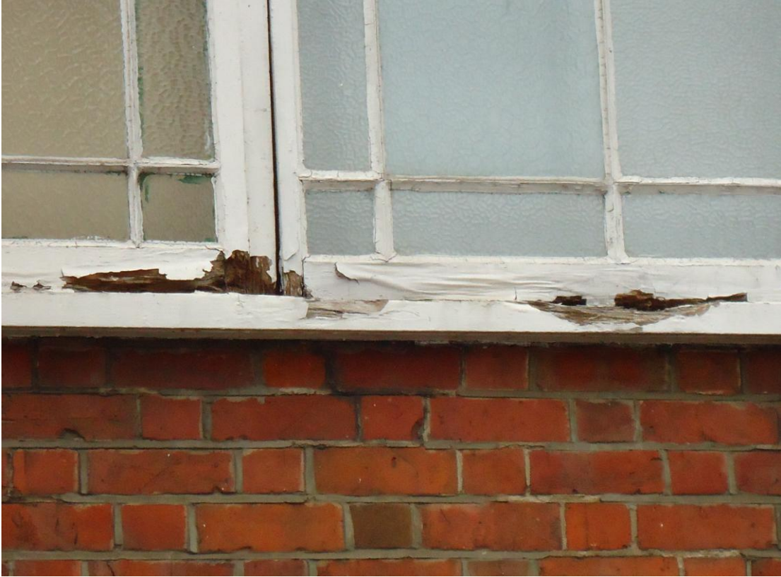
Extensive decay to East elevation covered walkway
