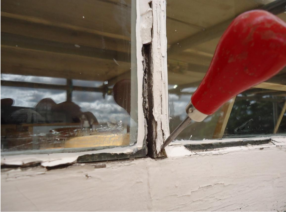
Decay to glazing bar and failed putty
