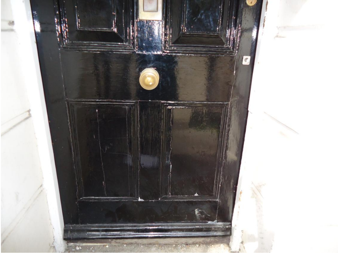
Splits in timber front doors
