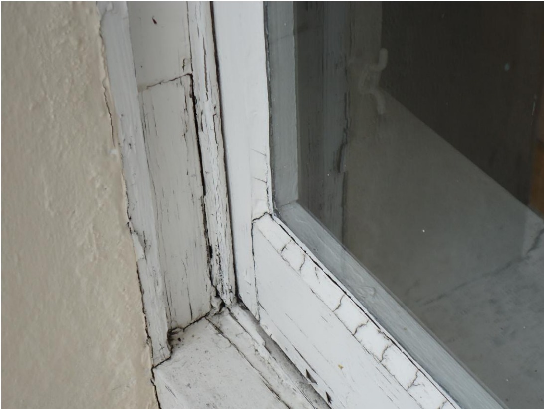
Example of failed putty, open joints and deteriorating paint
