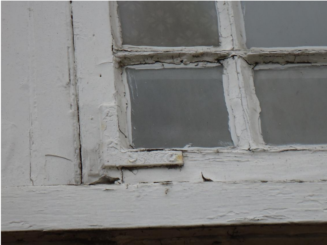
Failed putty, paint and a bracket used to repair a failed joint
