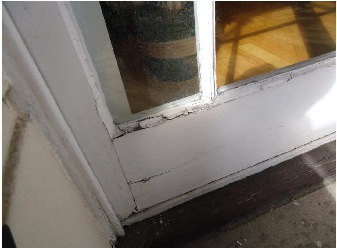
Open construction joint and horizontal split to the timber
