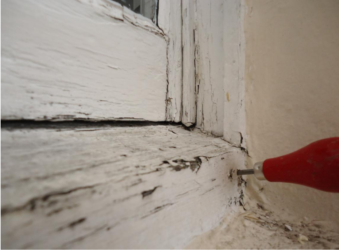
Decay to the cill, failed paint and an open sash construction joint
