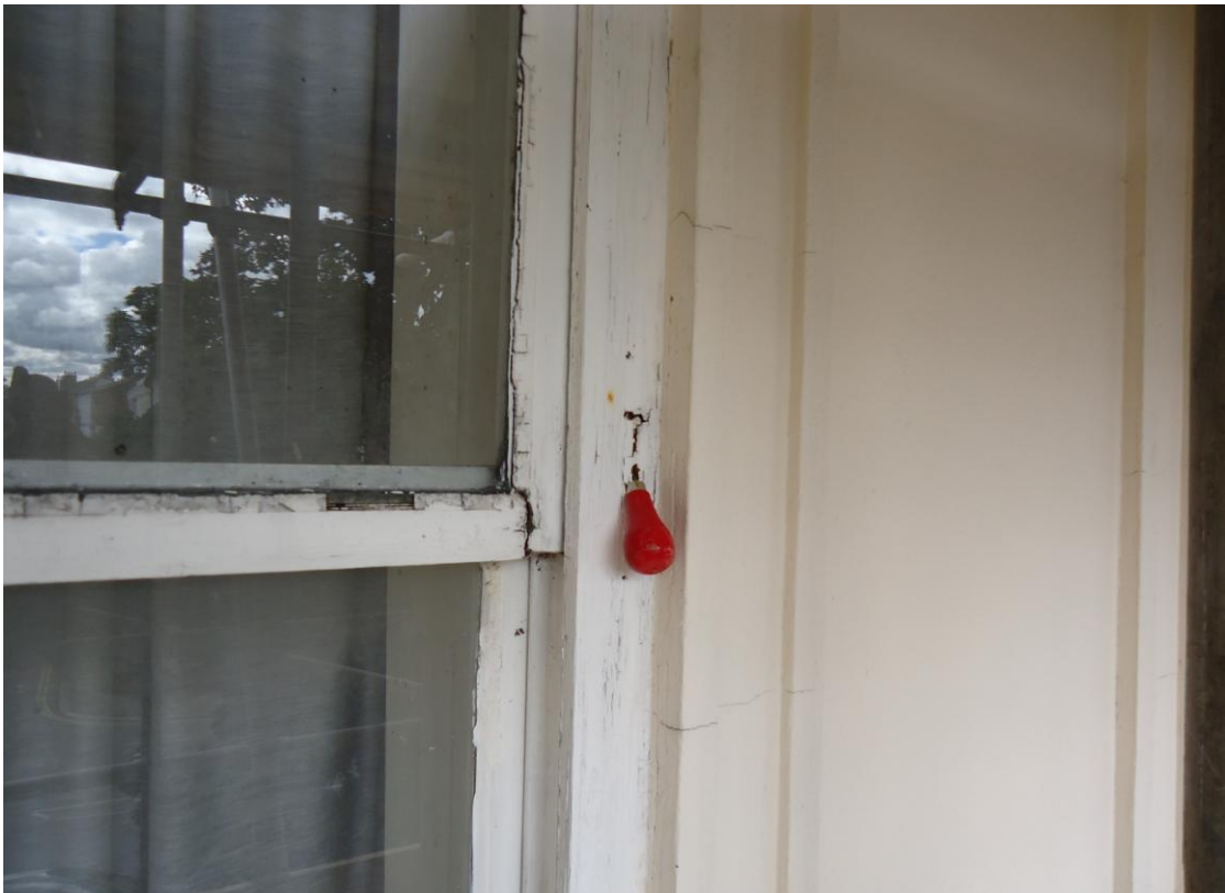
Decay to outer sash lining
