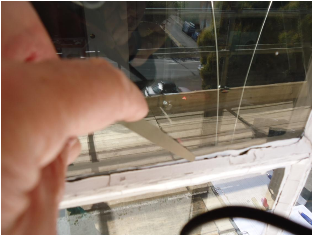
Gap between glass and putty allowing moisture ingress
